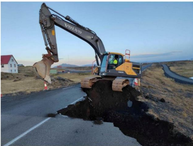
Streetworks continue after cracks emerged on a road due to volcanic activity near Grindavik, Iceland obtained by Reuters on November 14, 2023. Road Administration of Iceland via Facebook/ Handout via Reuters. TPX images of the day
