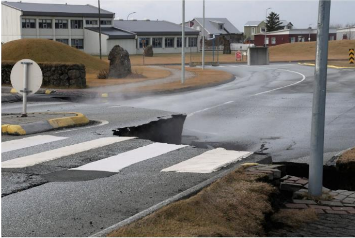
A road is damaged in the village of Grindavik, which was evacuated due to volcanic activity, in Iceland November 14, 2023. REUTERS/Ben Makori
