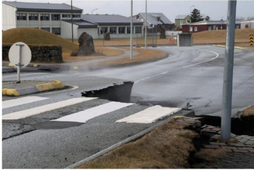
A road is damaged in the village of Grindavik, which was evacuated due to volcanic activity, in Iceland November 14, 2023. REUTERS/Ben Makori
